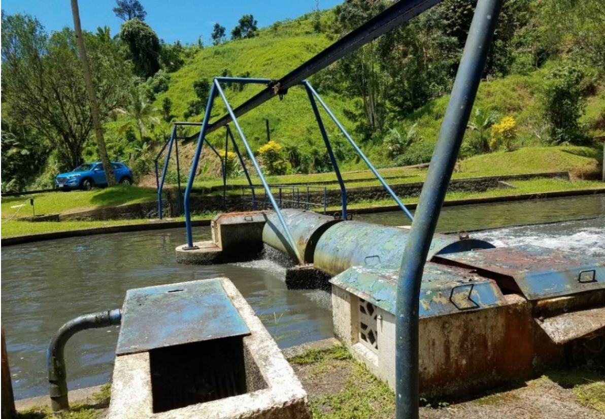
Figure 4: Oxidation ditch with surface aeration at Naboro WWTP
